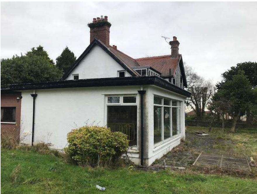
Existing felt roof has severe water ingress
