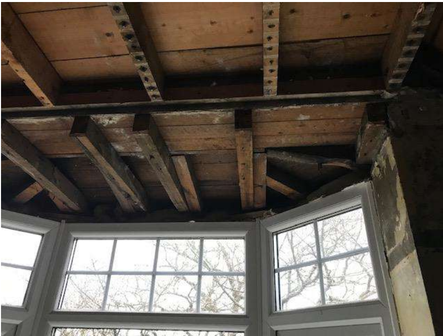
Flat roof and Upvc bay window at first floor level to Bedroom 1
